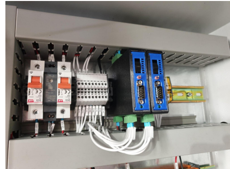
VibWire-301 in a PC Data Acquisition System
